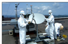
Installation in an evacuation zone.
